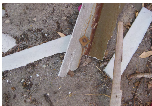
Figure 4 Broken ACM sheeting.
